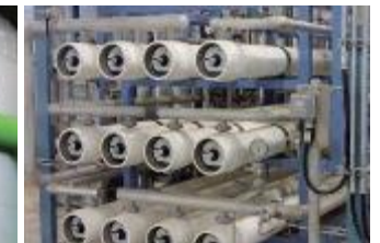
RO (Reverse Osmosis)
