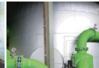
CPP (Condensate Polishing Plant)
